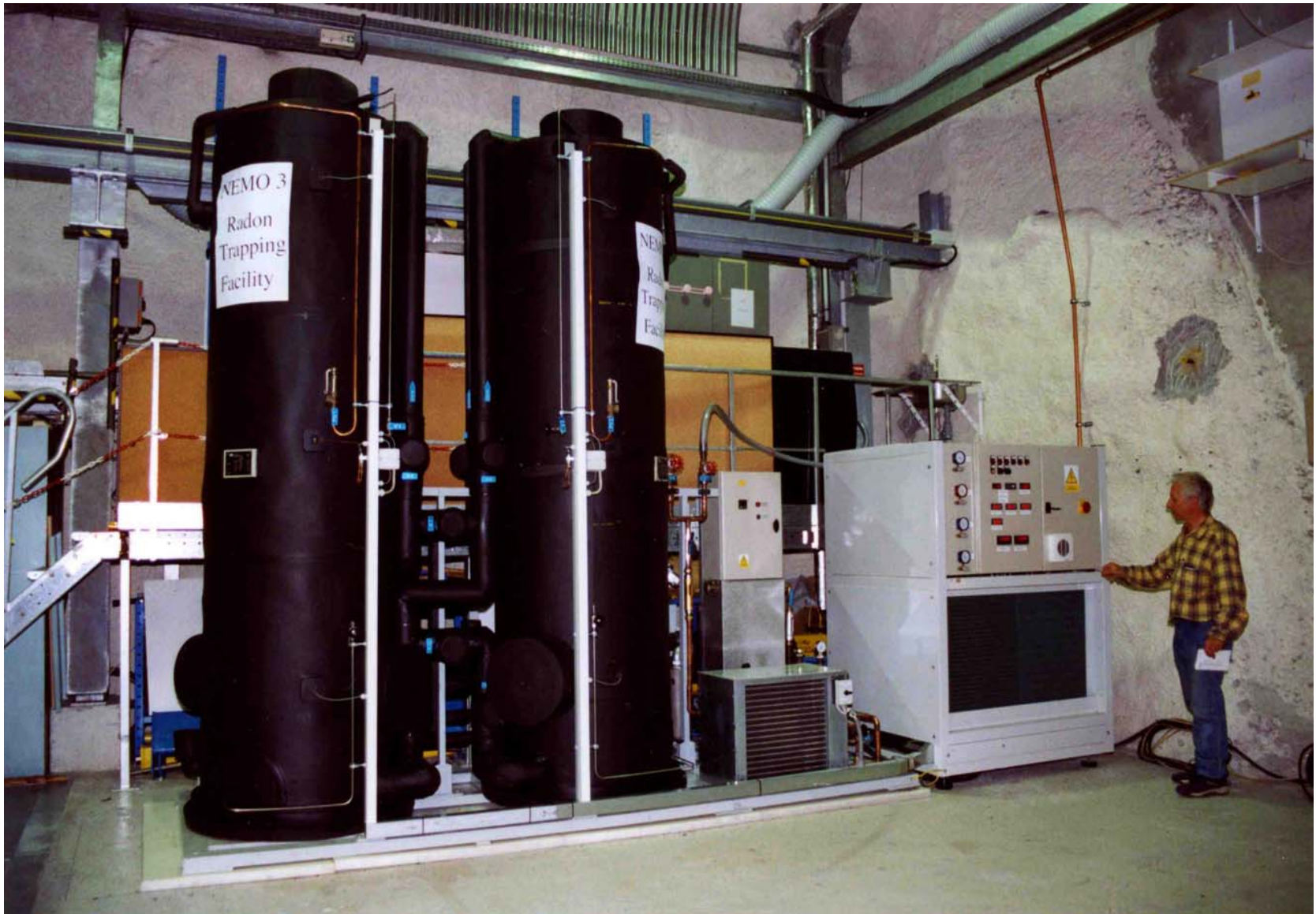
Anti-Radon Facility inside the lab
